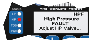
High Pressure Fault
