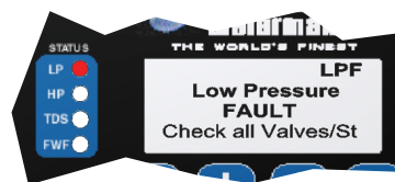
Low Pressure Fault
